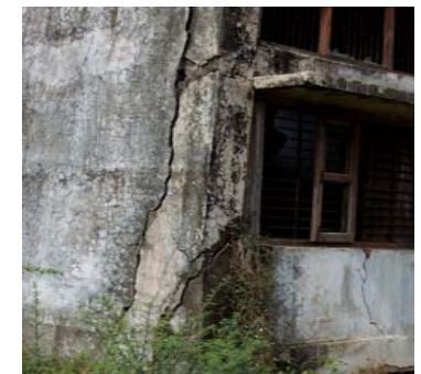
Cracked wall at ITI Ankleshwar
