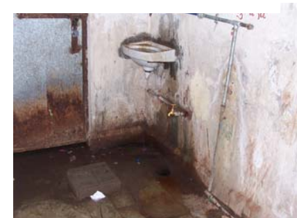
Location of drinking water facility at ITI Ankleshwar
